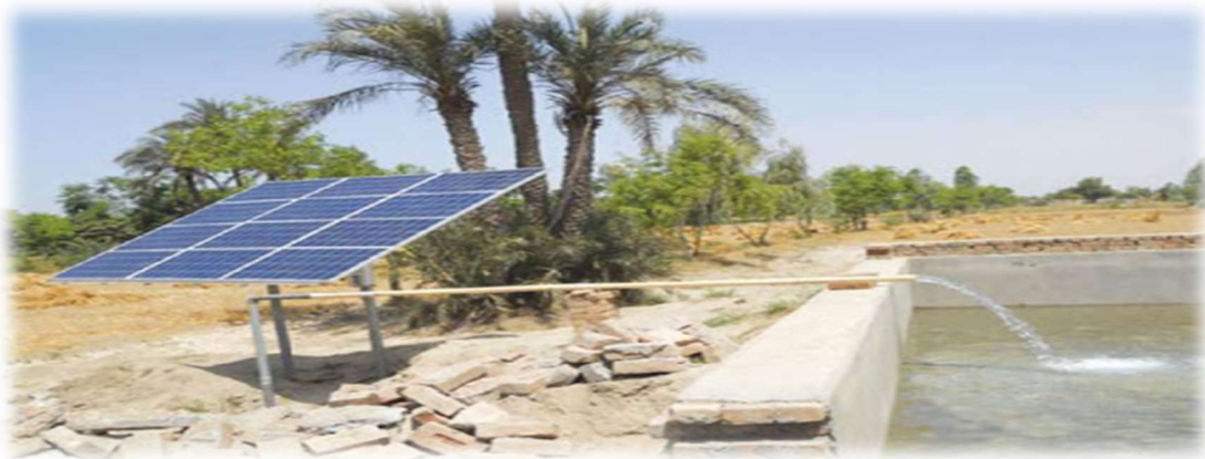
Figure 21: An image of Solar system in operation
